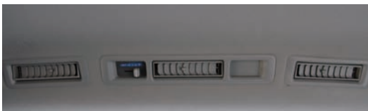
Rear air conditioner vent
